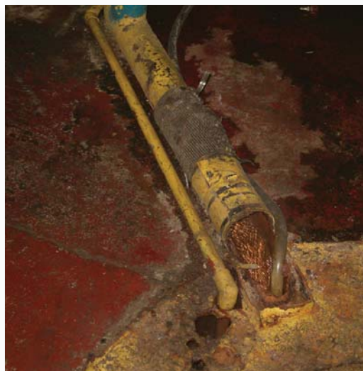
Tank overflow that cost $91,000 a year in chemicals, water and energy loss.
